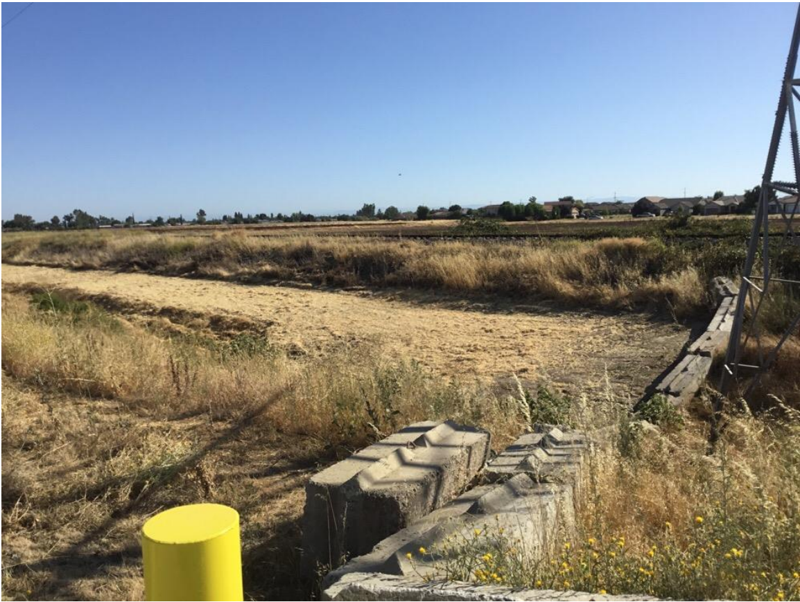
Photo 1: During this reporting period, construction crews completed gravel removal at Pull Site (PS) 1/13.
