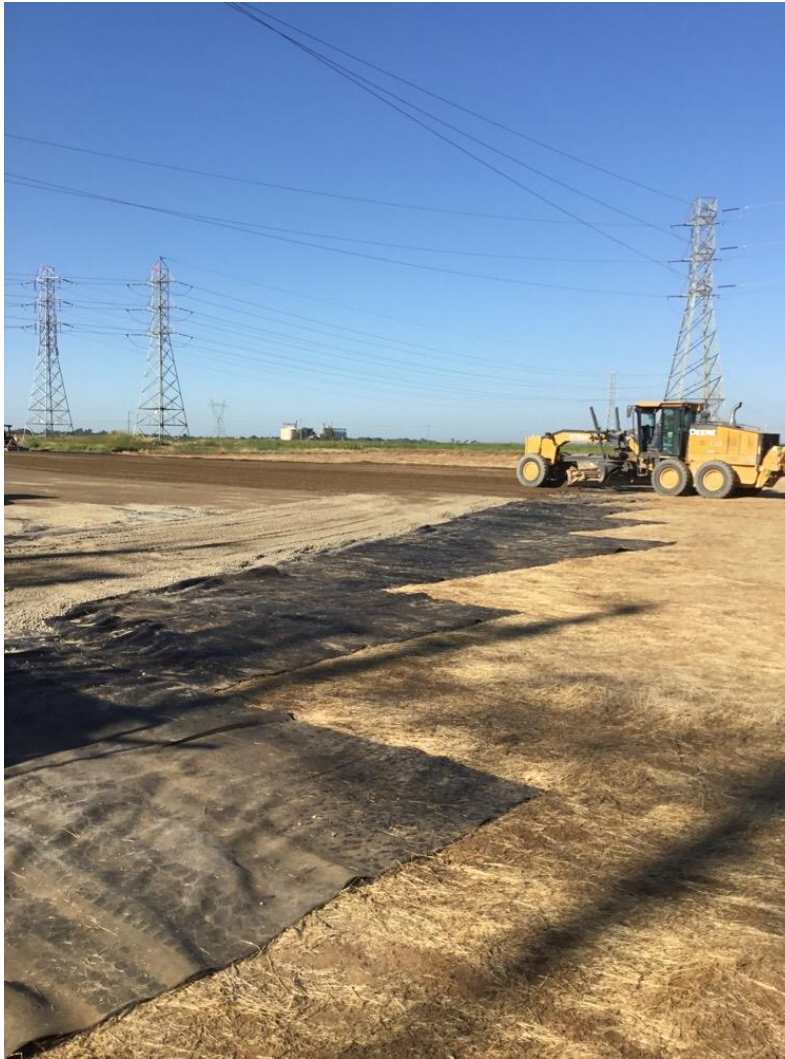
Photo 3: Grader spreading out gravel and rock material to winterize Landing Zone (LZ) 44/317.
